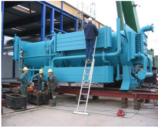
Figur 33: Absorptionsvarmepumpe under installation (Amager)
